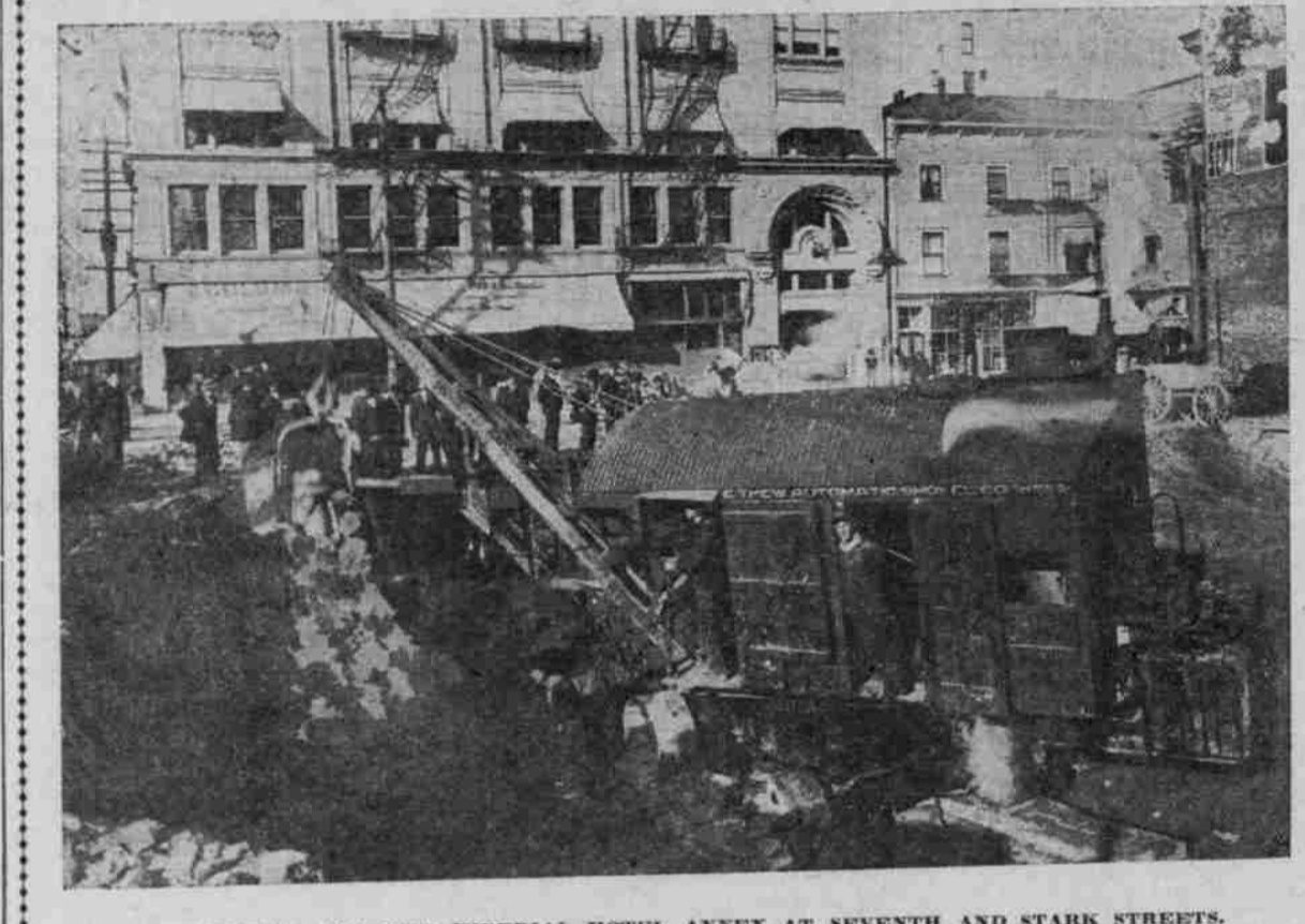
EXCAVATING FOR THE IMPERIAL HOTEL ANNEX AT SEVENTH AND STARK STREETS. The above illustration shows a steam shovel at work excavating at the site of the Imperial Hotel Annex at Seventh and Stark streets. This will be an eight-story building and is being erected by the owner, Theodore B. Wilcox.
