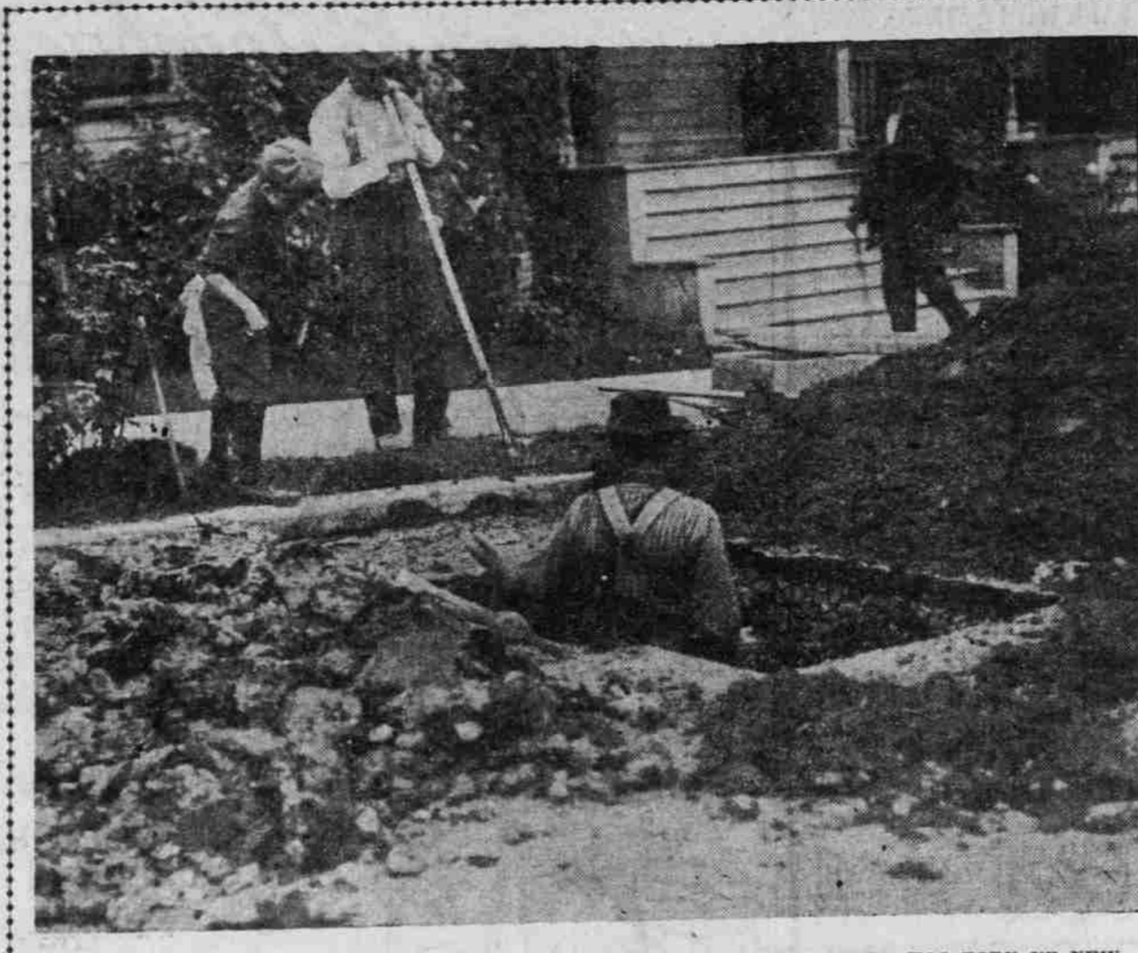
INTERSECTION OF TWELFTH AND ALDER STREETS, WHERE WATER BOARD HAS TORN UP NEW PAVEMENT.
