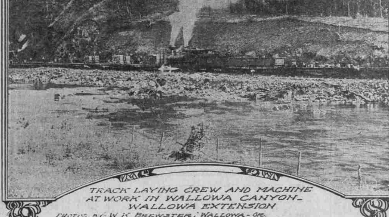
TRACK LAYING CREW AND MACHINE AT WORK IN WALLOWA CANYON WALLOWA EXTENSION PHOTO BY W. K. BREWSTER, WALLOWA, OR.
