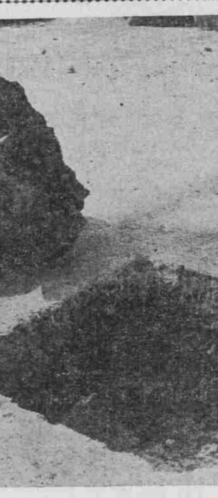
PHOTOGRAPH OF HASSAM PAVEMENT AT EAST SEVENTEENTH AND WASCOW STREETS, FROM WHICH CITY ENGINEER TAYLOR CUT A TWO-FOOT SECTION FOR INSPECTION BY THE COUNCILMEN.
