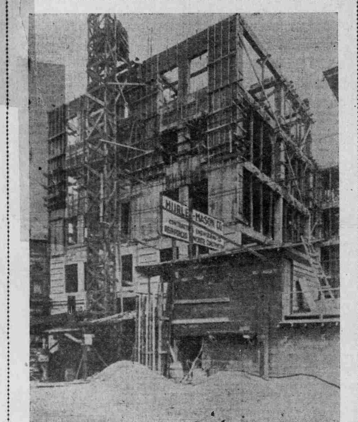
THE SEVEN-STORY ANNEX OF THE OREGON HOTEL, FACING PARK STREET, BETWEEN OAK AND STARK.
