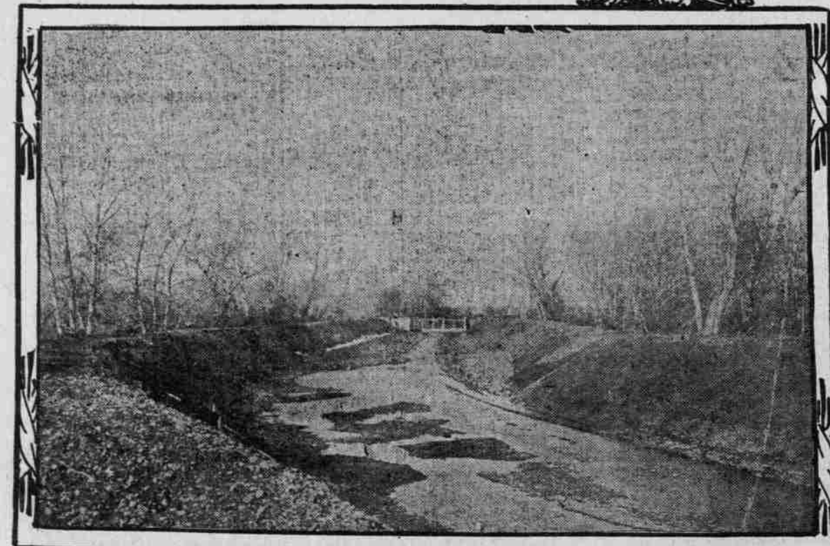
VIEW AT UPPER END OF FEED CANAL; LOOKING NORTH TOWARD REGULATING WEIR
