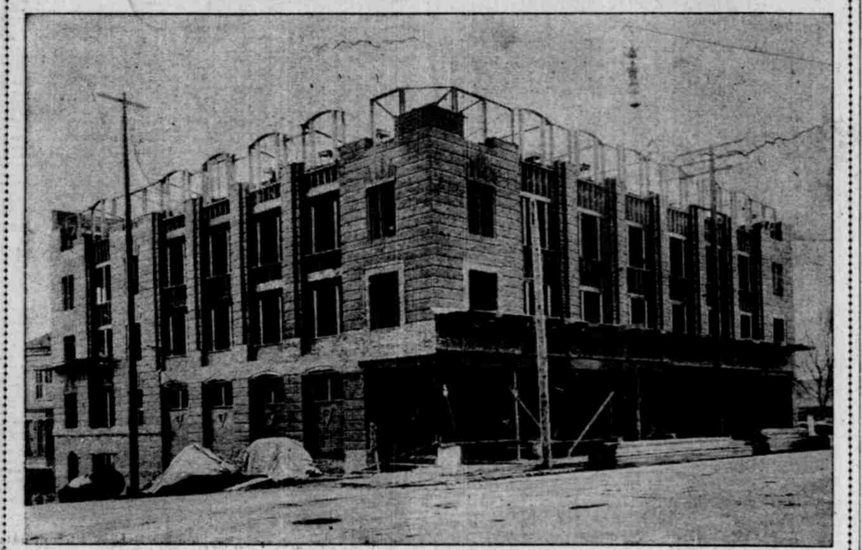
VIEW SHOWING PROGRESS OF WORK ON THE LAZARUS BUILDING AT FOURTEENTH AND WASHINGTON.
