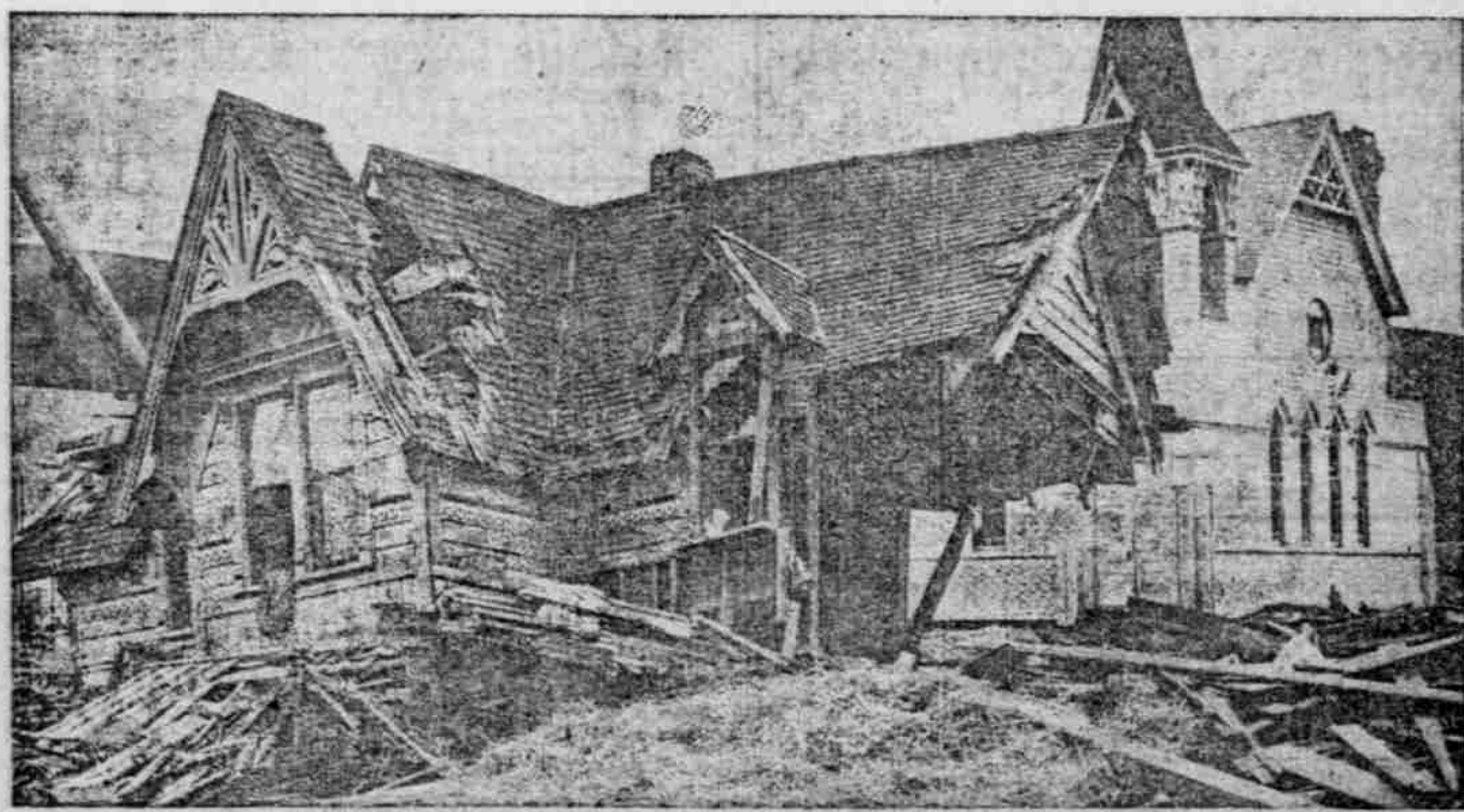
OREN MINOR'S DWELLING AGAINST M. E. CHURCH, ONLY BUILDING SURROUNDED BY THE WATERS THAT STOOD.
