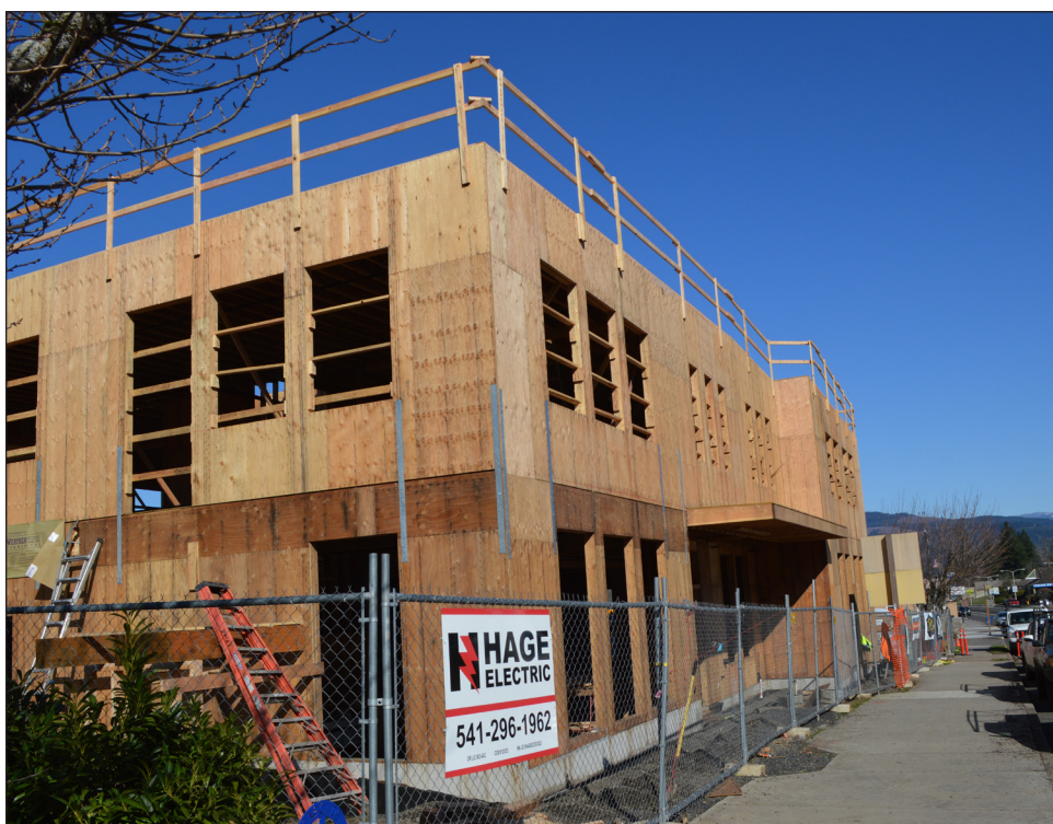
ON WANAPA Avenue in Cascade Locks, the walls are up on the new location for Thunder Island Brewing Company, scheduled for opening sometime this summer, according to co-owner Dave Lipps.
