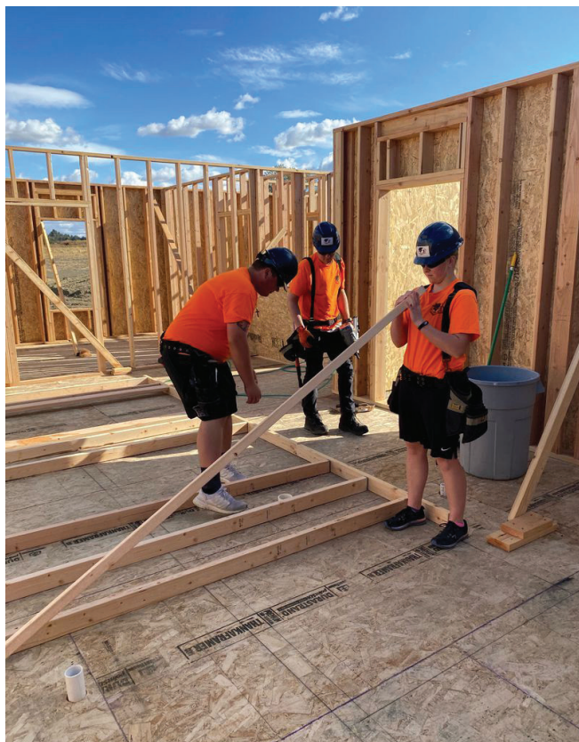
Columbia Basin Student Homebuilders Program Students help build a home in Hermiston.
