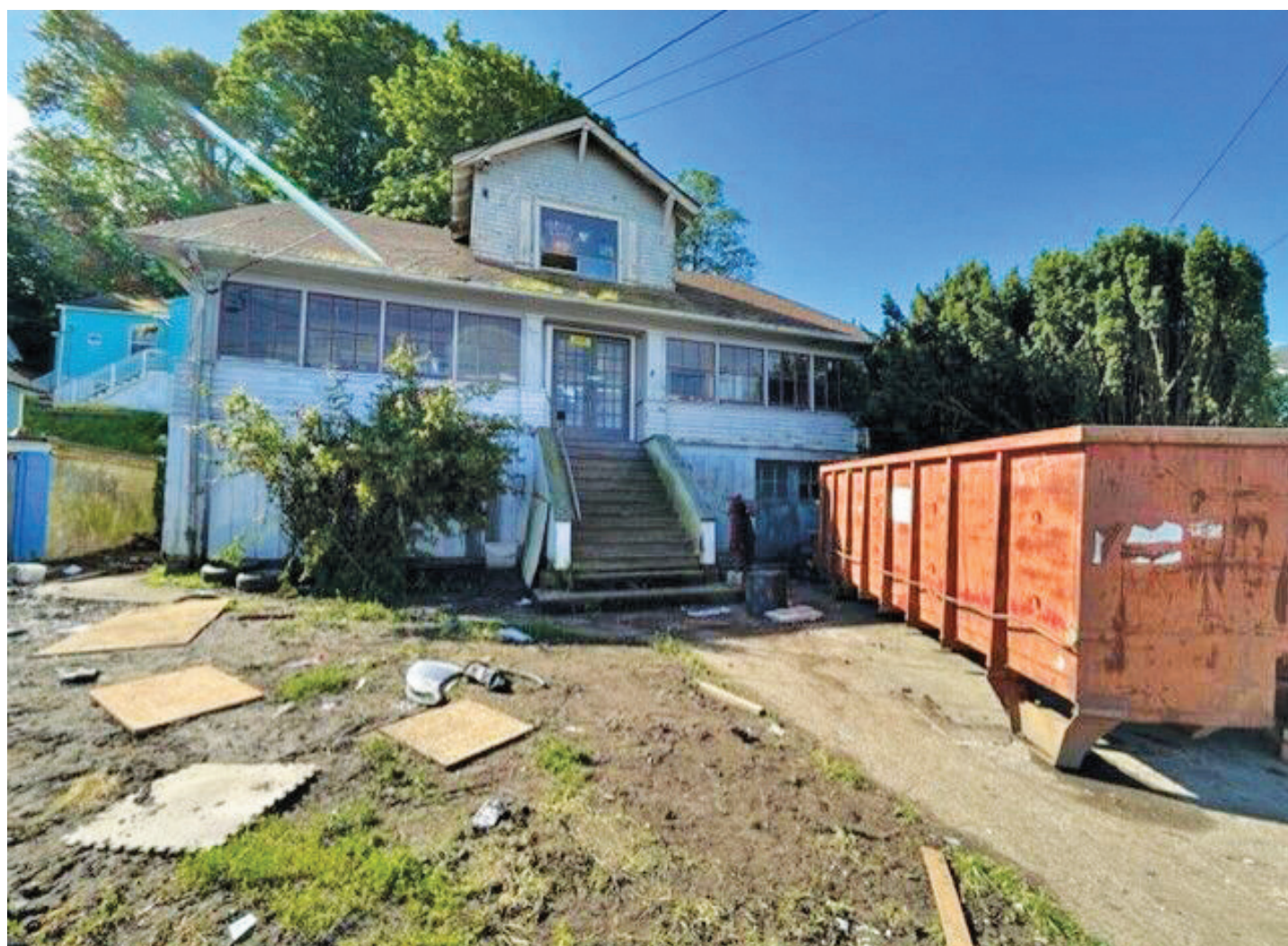
John Harper is restoring a house with a troubled history off W. Marine Drive.
