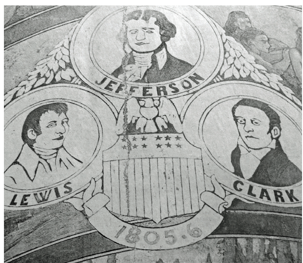
1972 – Several years ago, four lateral cracks appeared in the Astoria Column. Though they were fixed, they are still visible from the outside, running through parts of the mural.
