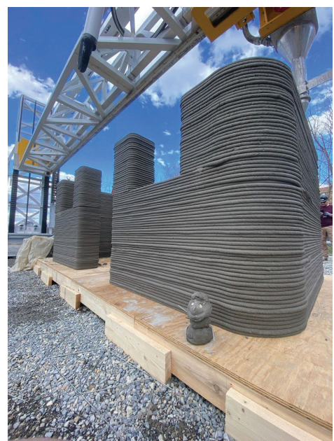
A structure printed with concrete and a 3D printer by manufacturer Alquist.
