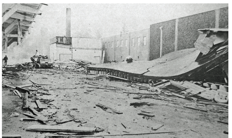
Modernization of the Point Adams Packing Co. in Hammond continued as workers demolished additional old structures on the firm's property in 1972.
