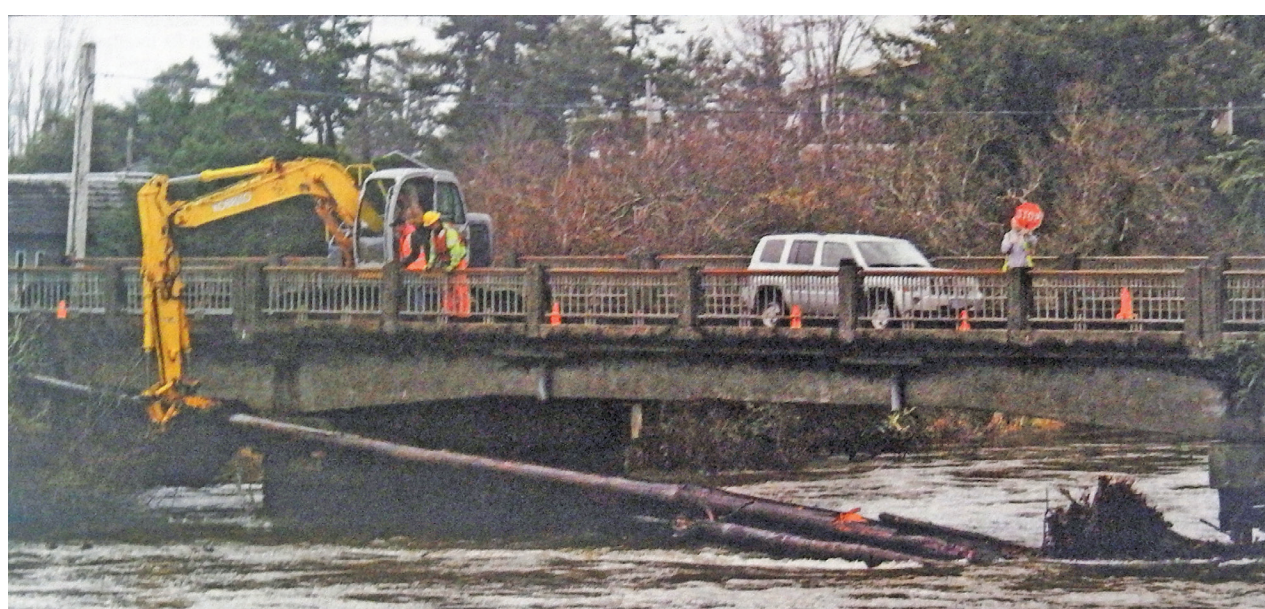
Workers use heavy equipment to remove a nearly 70-foot log in the Necanicum River resting against the Avenue U Bridge in Seaside in 2012.
