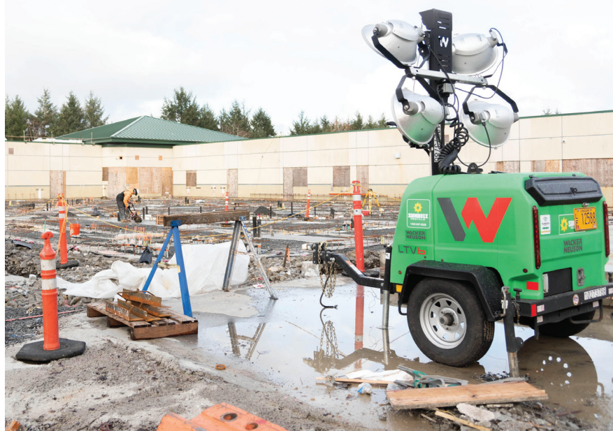
The new Clatsop County Jail is expected to be completed next year.
