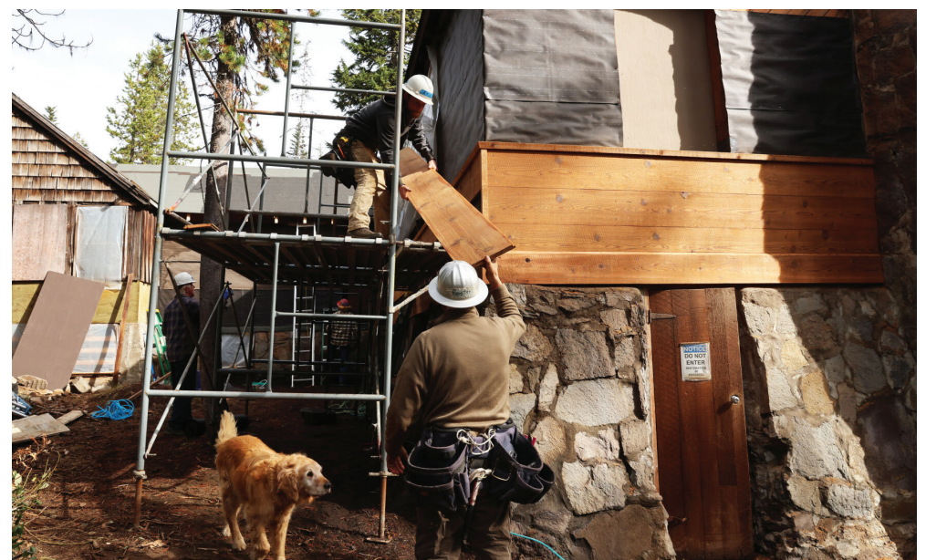
Bend resident Jim Redmond, a volunteer with HistoriCorps — a nonprofit historic preservation organization — hands a piece of siding to project supervisor Eric White in October while restoring the Santiam Pass Ski Lodge.
