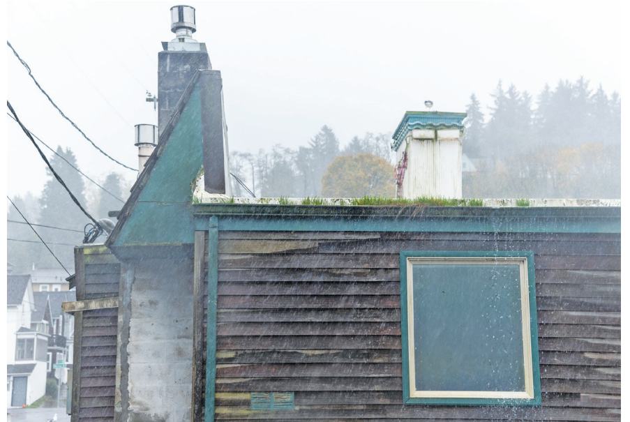
Rainwater rolls off the old Ship Inn restaurant, where a Fairfield Inn and Suites is planned.
