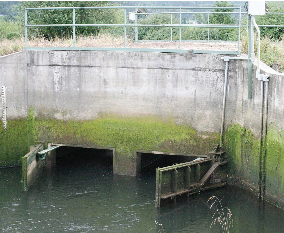
A tide gate at a dairy farm near Nehalem was installed in 2017 at a cost of $460,000, improving drainage and complying with fish passage rules.
