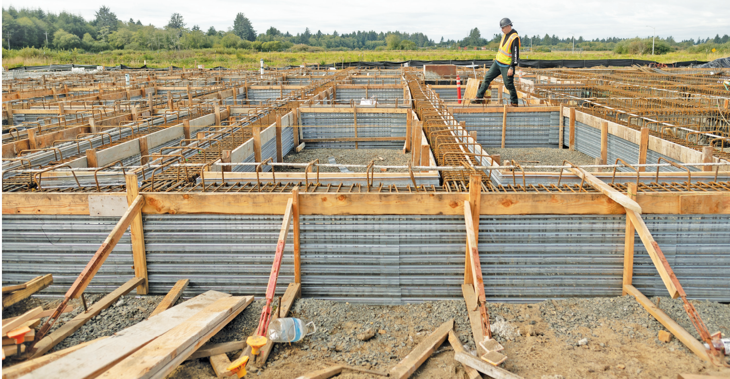
A new fishmeal processing plant has broken ground at the Astoria Regional Airport.
