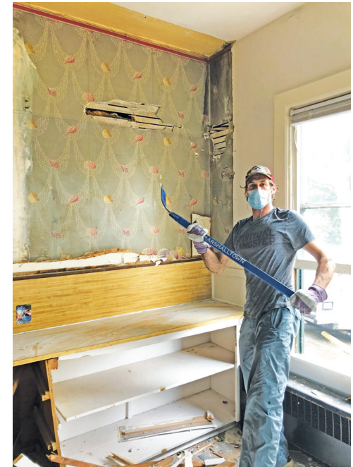
Djordje Čitović uses a crow bar to remove water-damaged walls in the Rosebriar.
