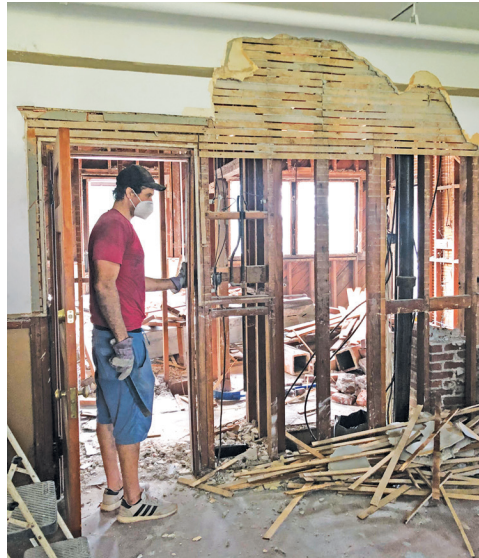
Djordje Čitović prepares to knock down a wall in the kitchen to open up the space.
