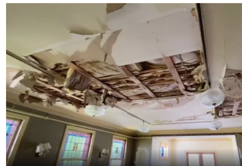
A leaking toilet created a massive hole in the chapel ceiling during the renovation process.
