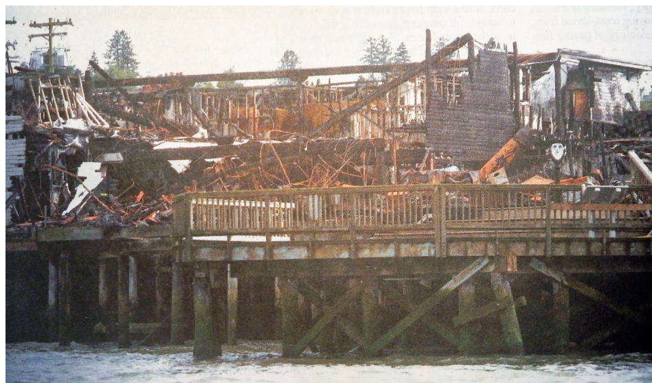
Rubble sitting atop the pilings at No. 10 Sixth Street and the Cannery Cafe in 2011.
