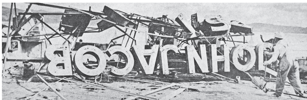
Workmen for Coast Marine Construction Inc. removed the John Jacob Astor Hotel sign from its precarious position atop the building in 1971. The sign had been twisted in a storm and was hanging partially over the side of the building.
