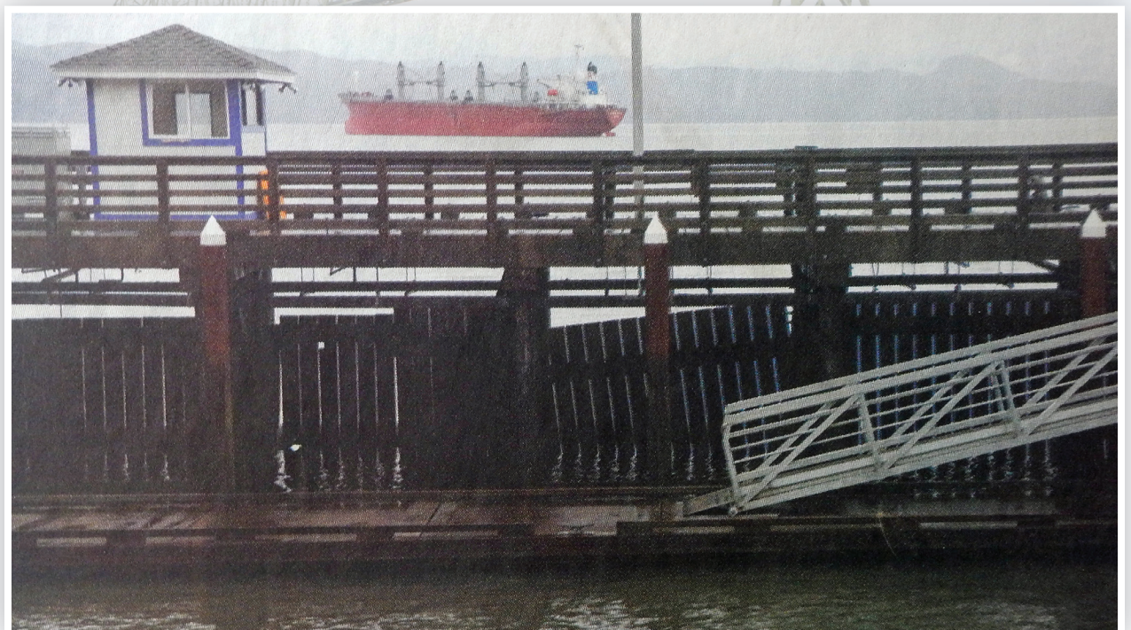
The 17th Street Dock required repairs in 2011 after years of deterioration.
