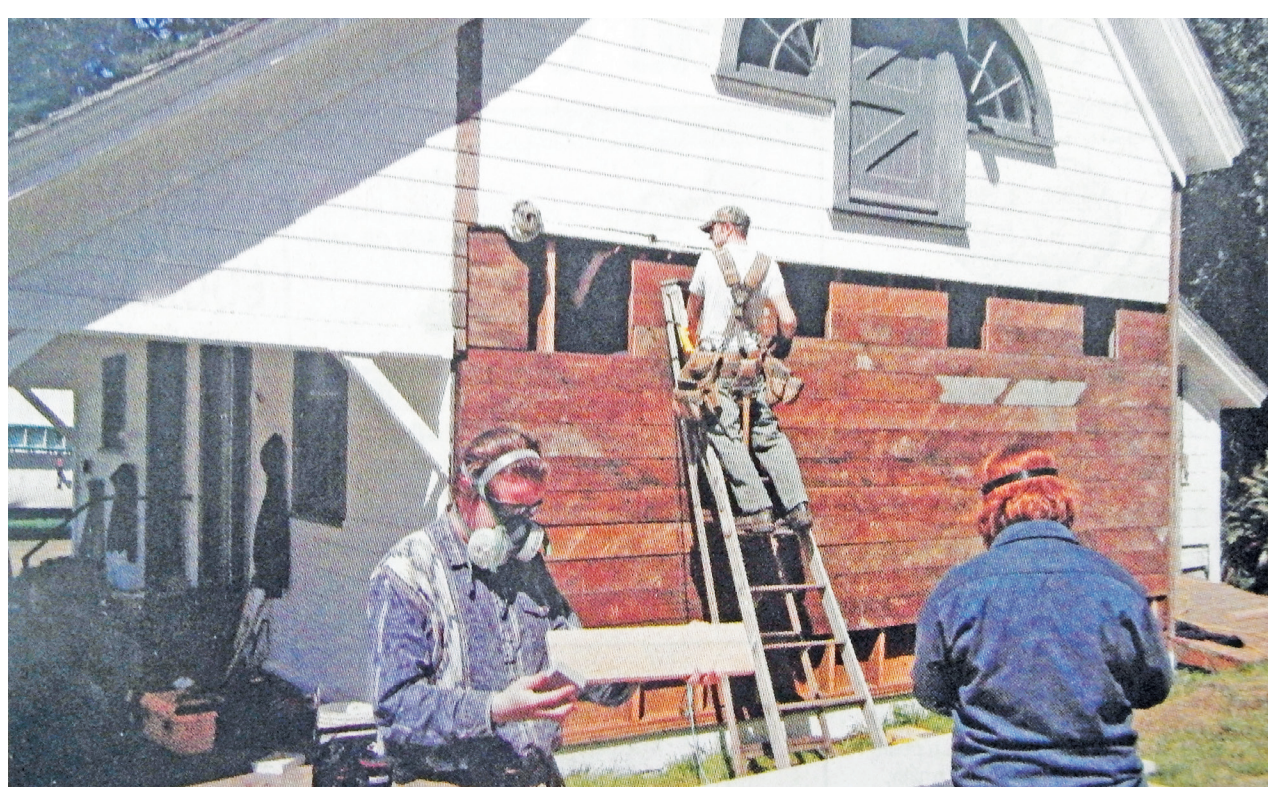
From left, Richard Balkins, Joseph Sakrisson and Larisa Zimmerman reconstruct two deteriorating sides of the North Head Lighthouse barn in 2011.
