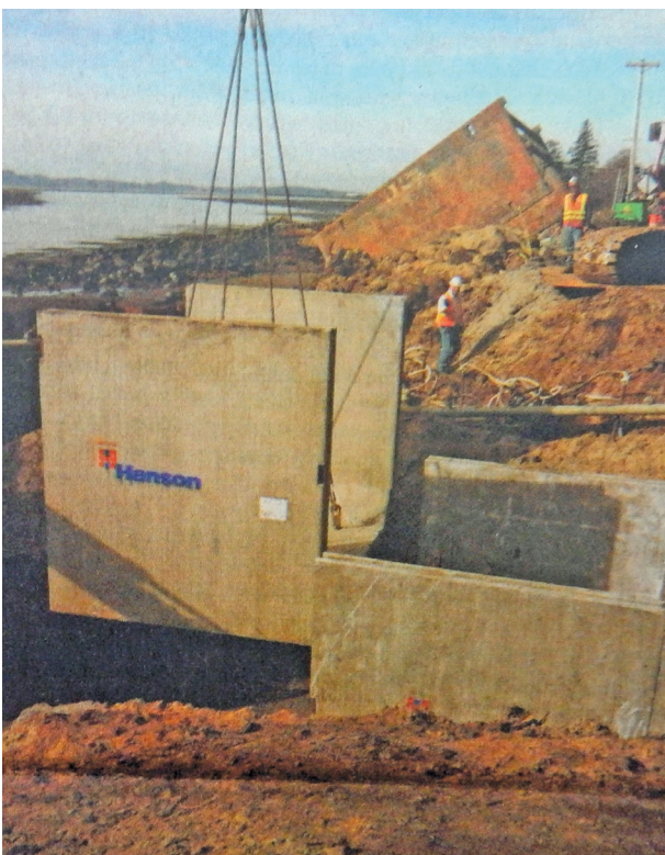
Sections of a 12-foot-wide culvert are installed beneath U.S. Highway 101 near Chinook, Washington, in 2011.
