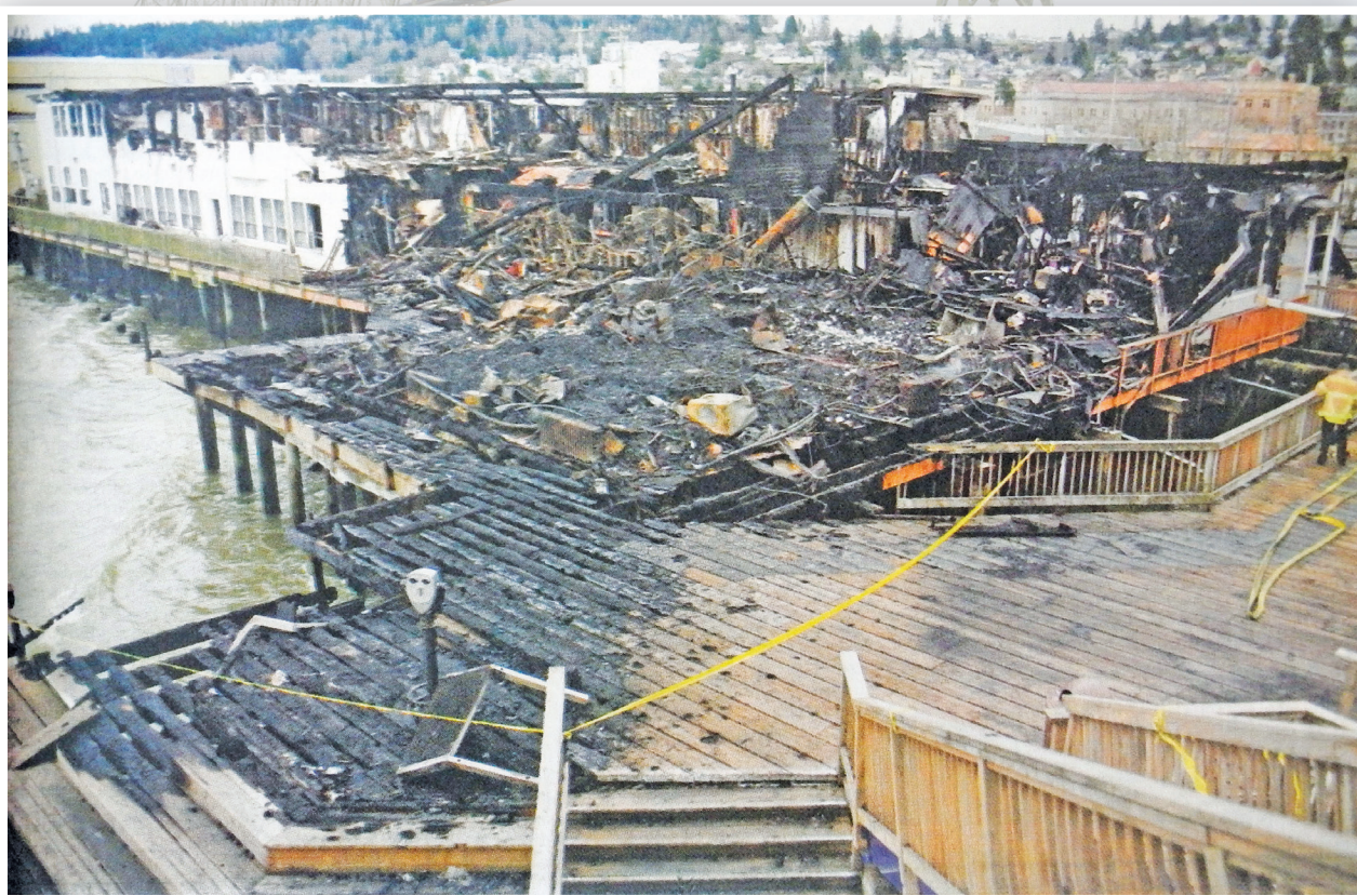
Rubble from the fire that devoured the northwest corner of the No. 10 Sixth St. building in 2010.
