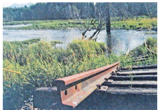
Water rushes in past the breached dike and disconnected railroad tracks at high tide at the Warren Slough in Knappa in 2010.
