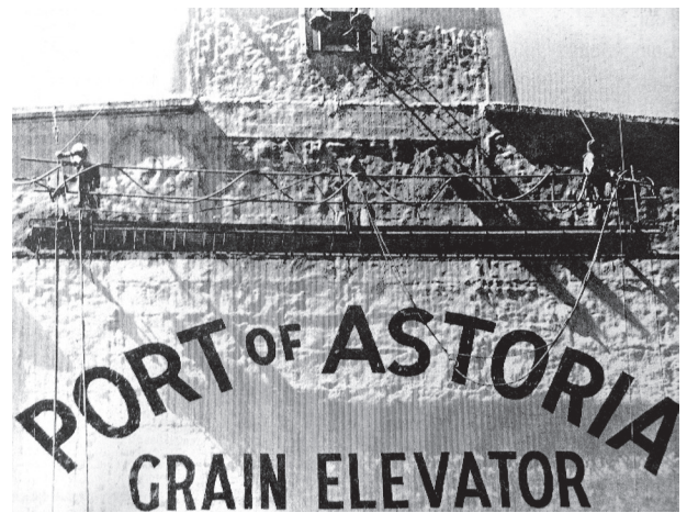
Workmen progress on refinishing the exterior of the grain elevator at the Port of Astoria docks in 1970.
