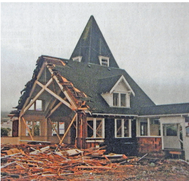
Only a portion of the old Our Lady of Victory Church building remained after demolition in 2010, making way for a new church twice the size on the same site on Ocean Way in Seaside.
