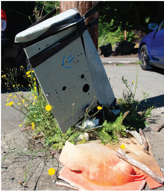
Hailey Hoffman/The Astorian The heavily-taped CenturyLink junction box sits off of U.S. Highway 26 surrounded by trash, weeds and a destroyed traffic cone.
