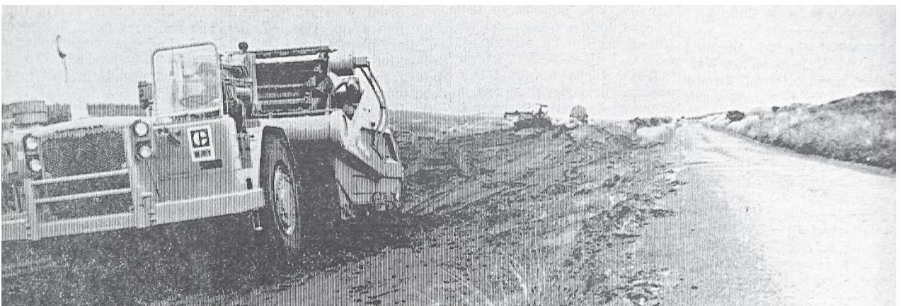
Construction West works on construction of a new road from Battery Russell to the South Jetty at the Columbia River entrance in 1970.
