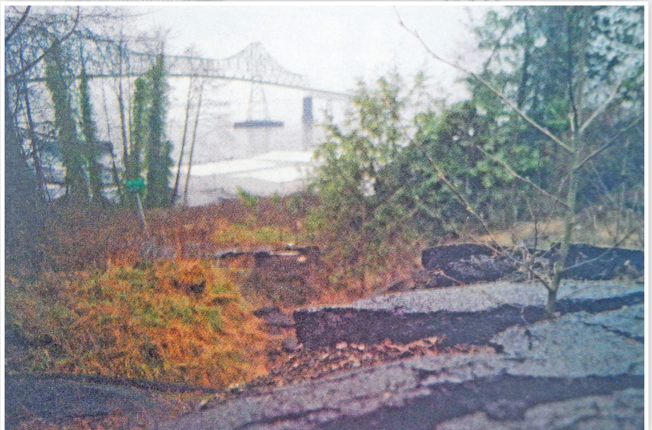
A tree grows from cracks in the pavement near the corner of First and Commercial streets in 2010. The Astoria City Council is considering creating a pedestrian trail from Duane Street to Commercial Street.
