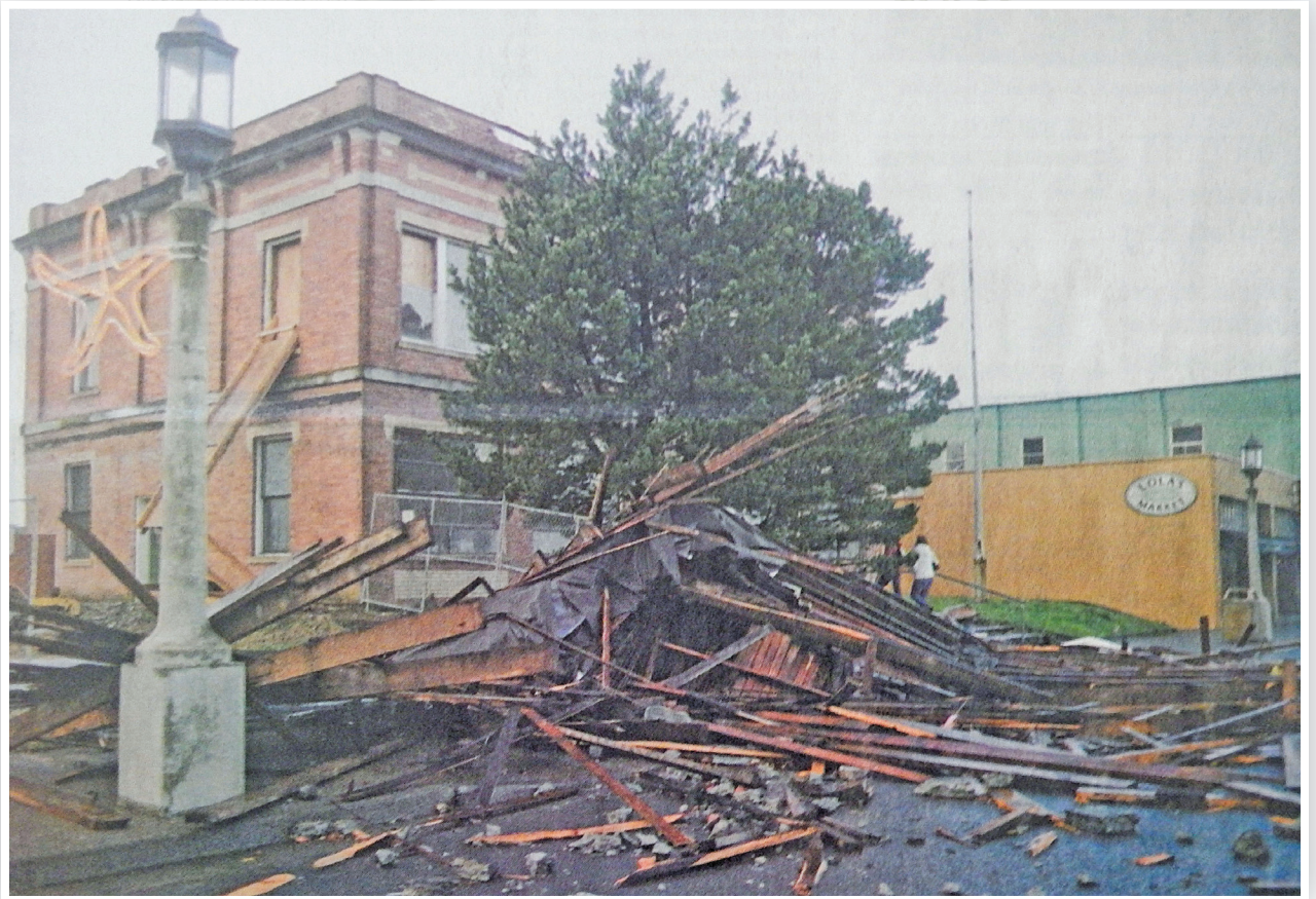
The roof of the old Seaside City Hall at 859 Broadway littered the sidewalk and street after being blown off by high wind overnight.
