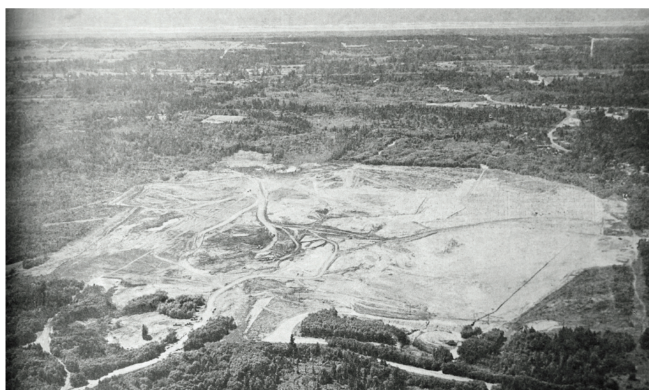
The site preparation work at Northwest Aluminum in Warrenton took over a year to complete. The silty clay soil could not be worked when it was wet, and an unusually wet year caused many delays.
