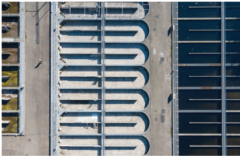
After salmon eggs are spawned, they are released into larger ponds outdoors to grow. Over the course of decades, the concrete walls and flooring has corroded.
