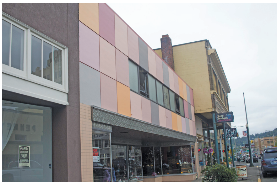
William Hicks, who purchased and redeveloped the former Abeco Office Systems store on Commercial Street into a minimall, recently removed the tin facade and replaced it with a more colorful covering.
