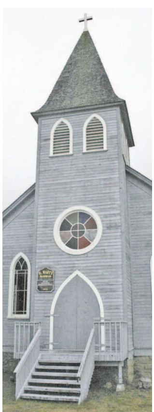
St. Mary's McGowan Catholic Church is in need of repairs.
