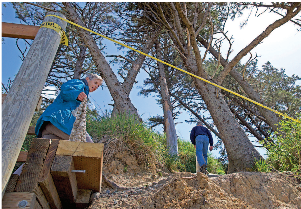
Connie and Joe Ratti climb their way up the damaged trail leading to the parking lot at Arcadia Beach.
