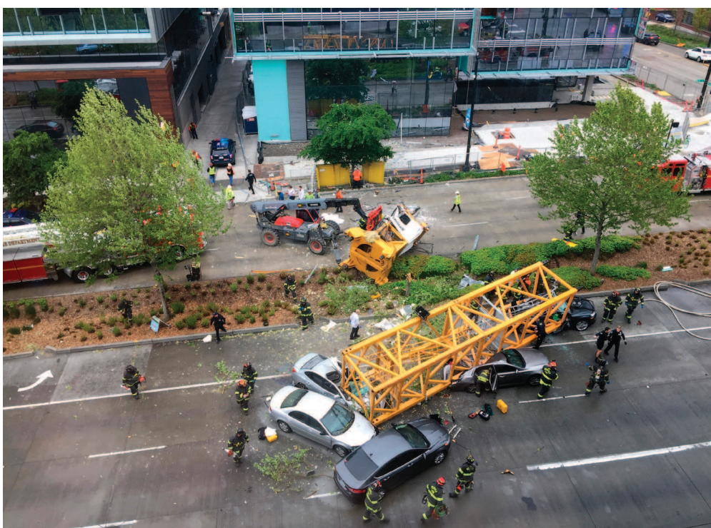
AP Photo/Frank Kuin Fire and police crew members work to clear the scene where a construction crane fell Saturday from a building on Google's new Seattle campus.
