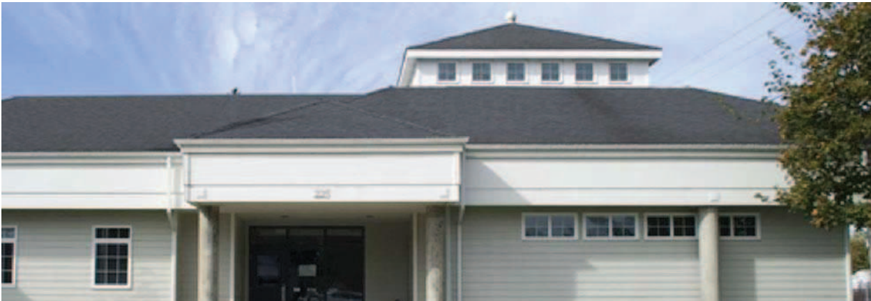
The roof at Warrenton City Hall needs repairs.
