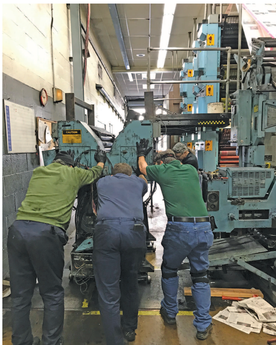
Daily Astorian press crewmen Carlos Anaya, Clark Verd, Carl Earl and Jim Stanovich push out an old 2-1/2 ton black ink only press unit after removing it to make room for the new full-color 4-high tower.
