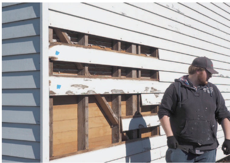
Students evaluate and make repairs at the replica of the historic Custom House in Astoria in 2018.
