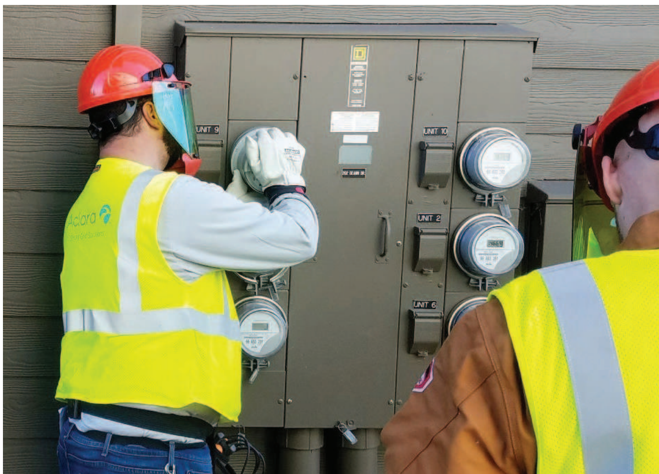
Pacific Power Installers with manufacturer Aclara Technologies will visit homes around Clatsop County starting in February to install Pacific Power's new smart power usage meters.
