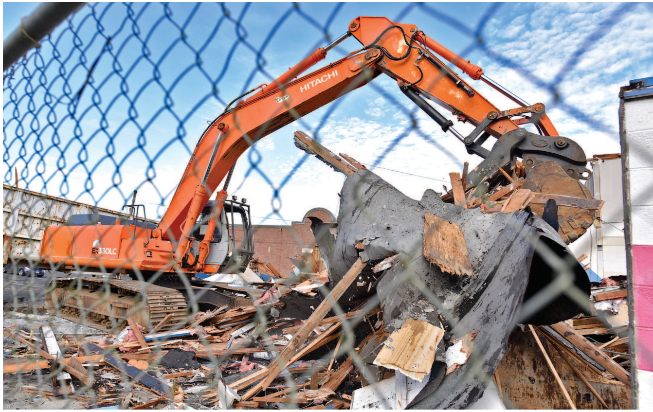
Heavy equipment is used to demolish the North Coast Auto Service building.
