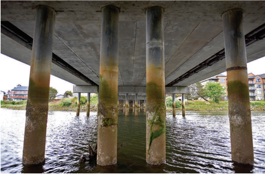
Several bridges and roads in Seaside have been deemed potentially problematic in an earthquake and tsunami.
