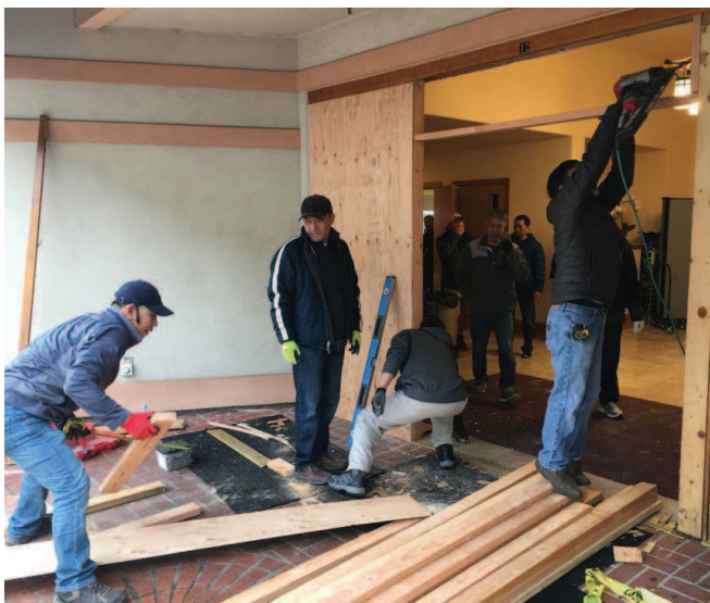
Shane Dixon Kavanaugh/The Oregonian Our Lady of Lavang, at Northeast 54th Avenue and Alameda Street, was extensively damaged on Monday after police say a driver plowed into the building.
