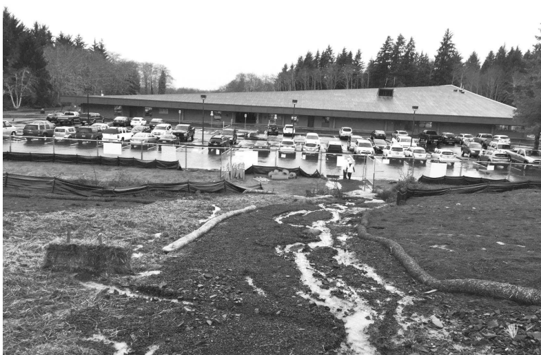
Heavy rains test mitigation measures at the campus.
