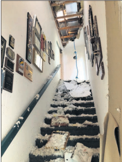
Hurricane damage at the Paul Brent Gallery in Panama City, Florida.
