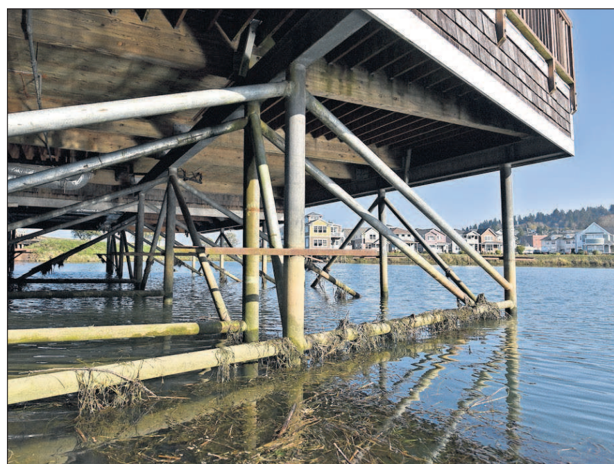
Structural elements support a home built over the water in Mill Pond Village.
